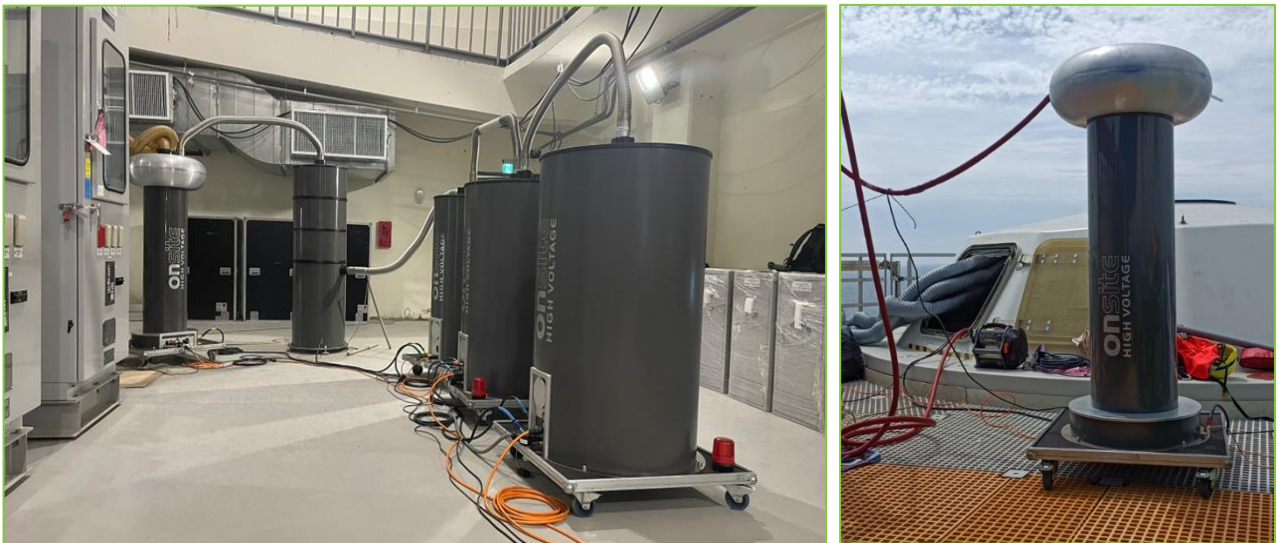
Export cables testing using DAC 300 kV system: Master unit with High-Power installed on the on-shore substation (on the left) Slave unit with Dual-Side installed on the off-shore substation (on the right)
