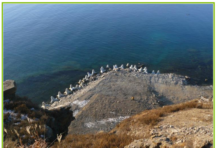
Transition point of 220 kV cable from land- to submarine. During the after-laying test by PD monitored DAC testing within the recommended power frequency testing range (20 Hz-300 Hz) PD activity has been detected and localized in one phase at a joint position (land part)
